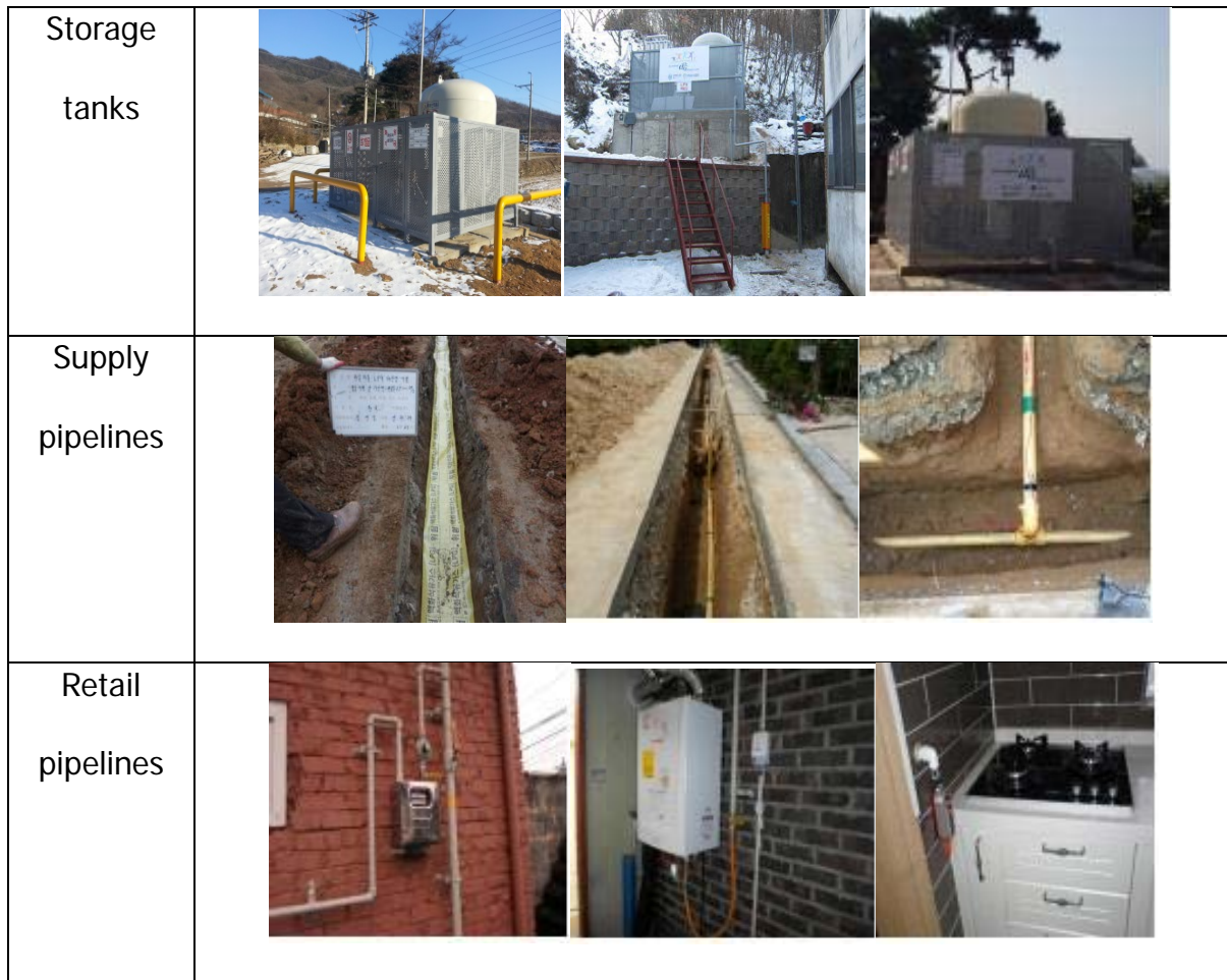
Figure 113. LPG storage tanks, supply pipelines and retail pipelines.
